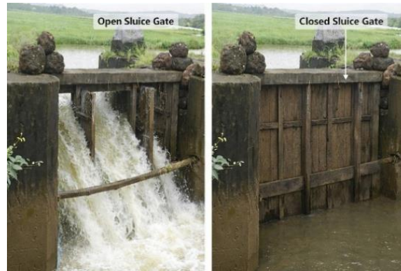
Figure3: Sluice Gate (Manos)
